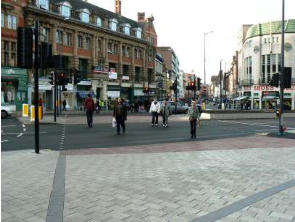
Super crossing at the junction of Granby Street and St Georges Way funded by Growth Point Funding and ERDF (European Regional Development Funding) - work completed 2010, resurfacing to road, new block paved footways, and controlled crossing.
