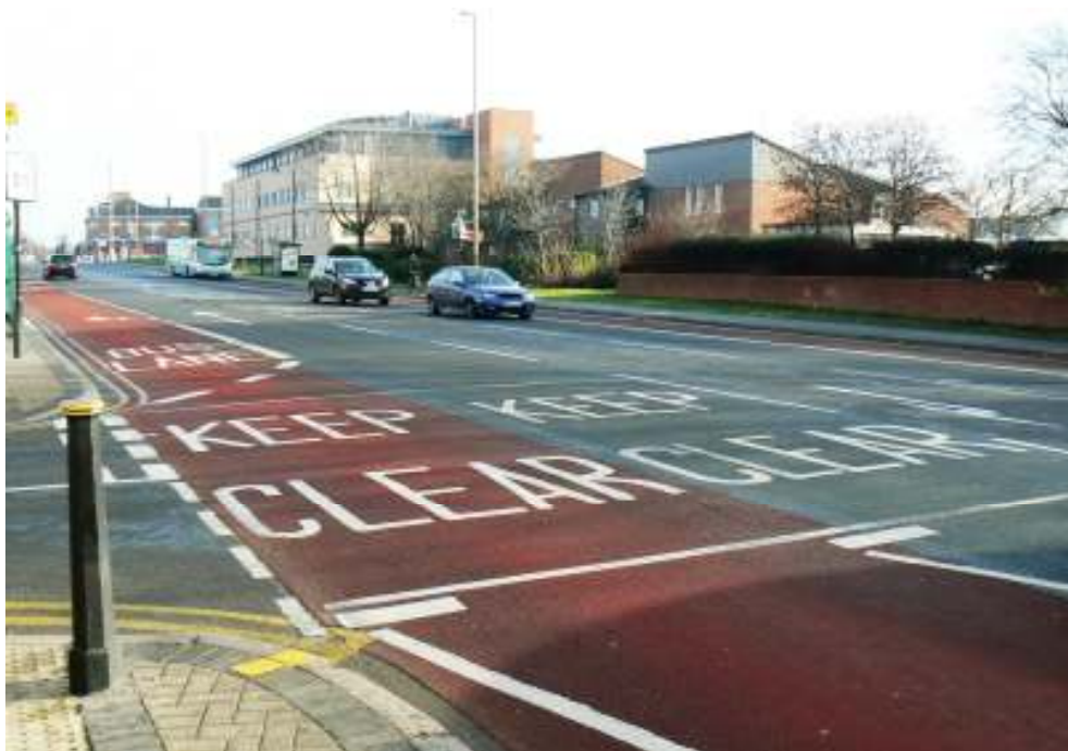
Integrated transport project on Humberstone Road (A47) completed 2010, resurfacing to road and footways, new bus lane and new anti-skid surfacing
