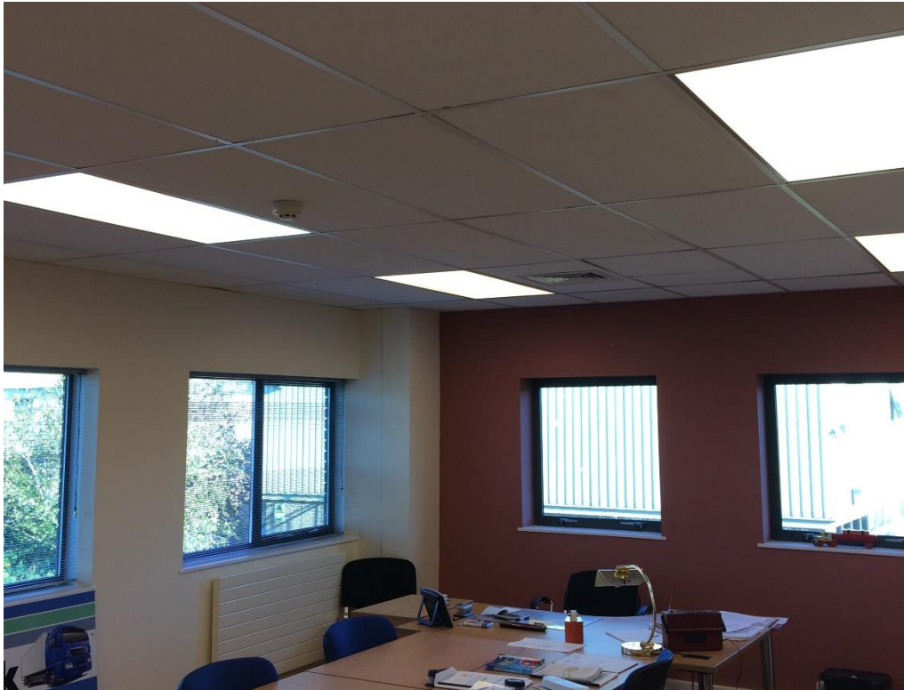
Above: LED lighting installed at Bakers Waste Services Ltd
