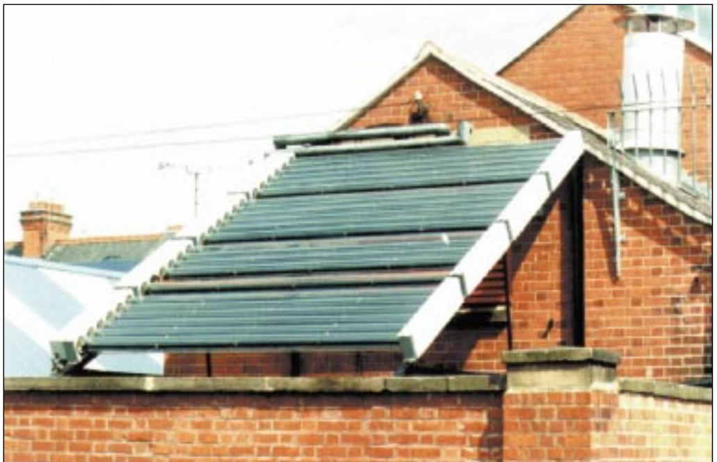
Roof-mounted Hitachi evacuated-tube collector at Cossington Street Sports Centre
