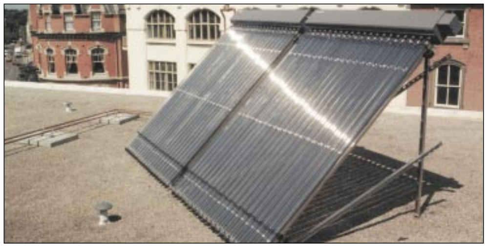
Solar collector on the roof of Phoenix House
