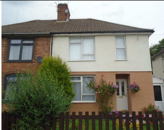
EWI finished with half brick slip and half plain smooth render above.
