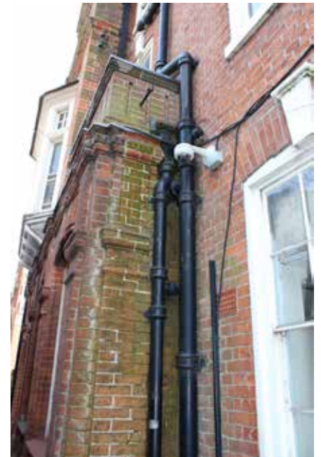
Example of cluttered frontage and stained brickwork
