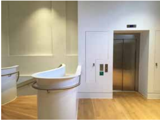
Lift (First Floor)
