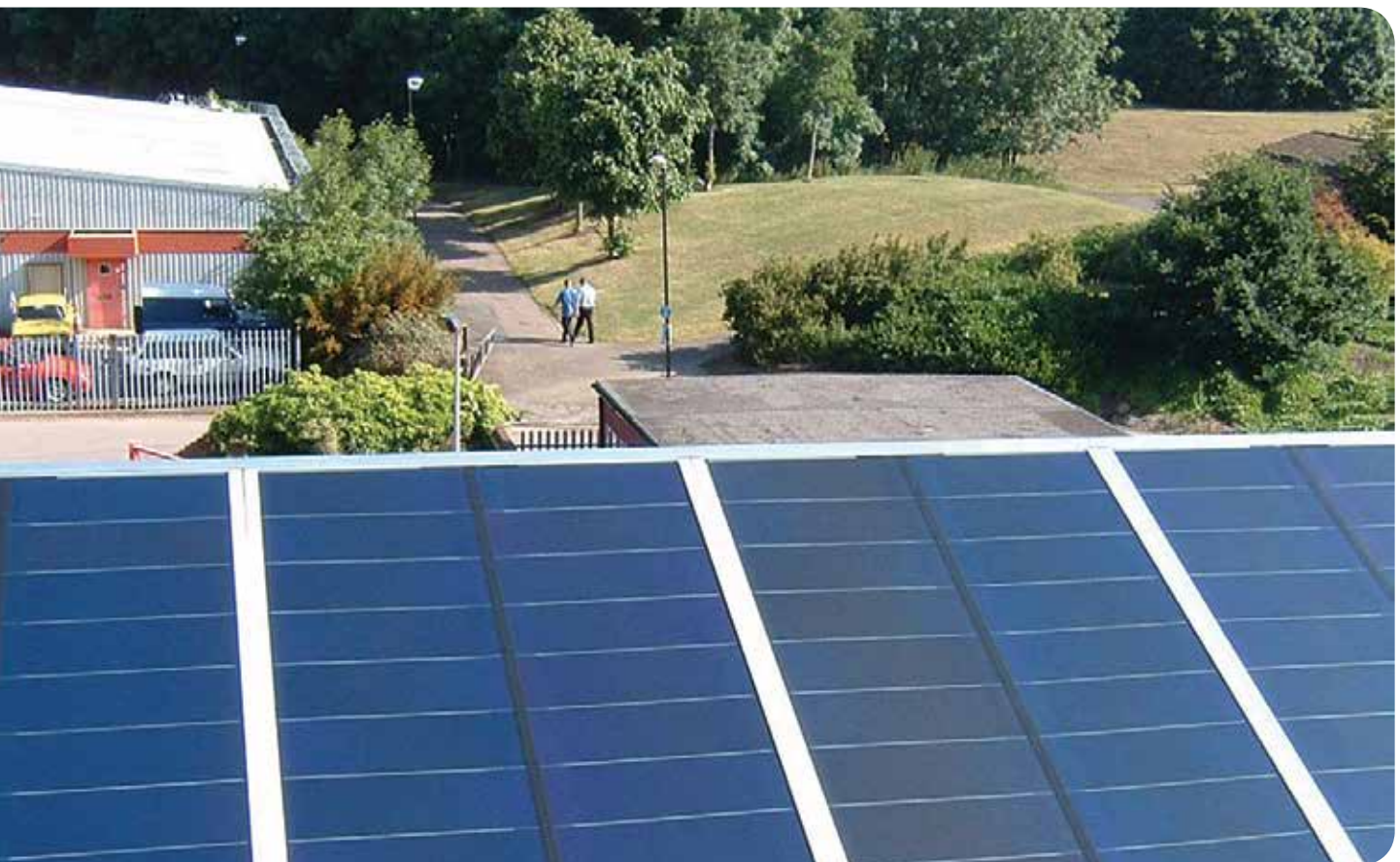
Solar panels on a roof
