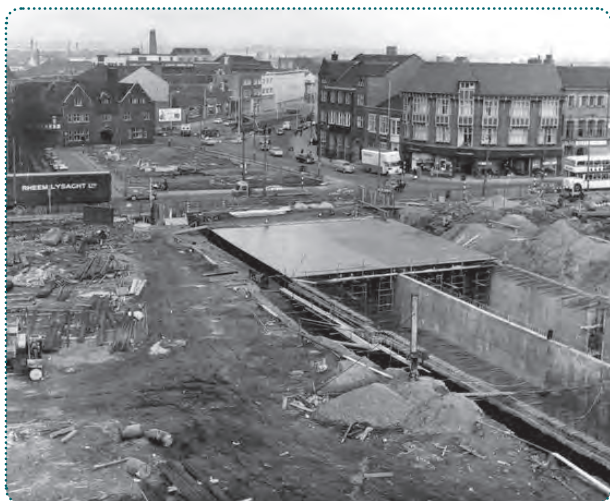
Figure 9: Underpass Construction in the 1960s - Many of the Adjacent to Southgates Blocks had been cleared. (Leicester Mercury)
