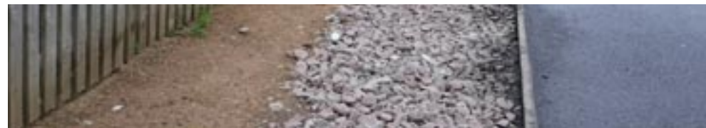
Water from car park entering filter drain and then to Swale. ASDA Leicester
