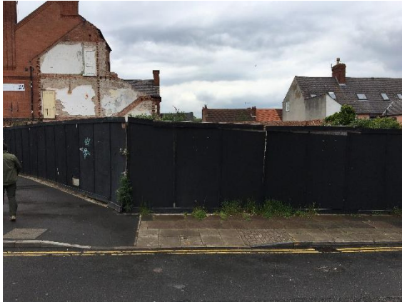
Figure 1: Vacant site at the junction of Carlisle Street and Hinckley Road was demolished in spring 2018.
